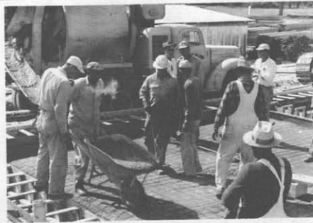
CONCRETE TRUCKS ON ISLAND KEPT BUSY: Here one of the trucks from the Island concrete plant prepares to unload concrete for the foundation of the operations building of the radar site.
