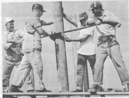
Pilings being leveled on the home of Mr. Fred Taegert by Mr. Bob Chasen's crew.
